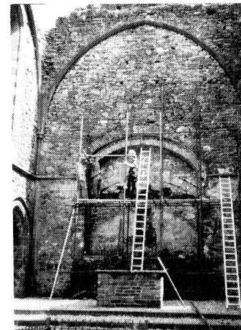
1980 East wall reinforced and pointed. Memorial altar to Fr. John Windle installed
