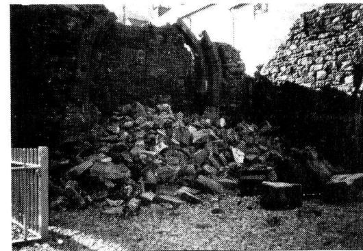
1984 A setback - wall collapse in the SW corner - repaired later that year
