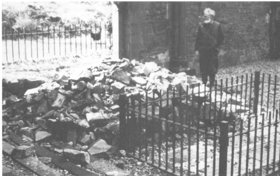
The latest wall collapse - December 1987
