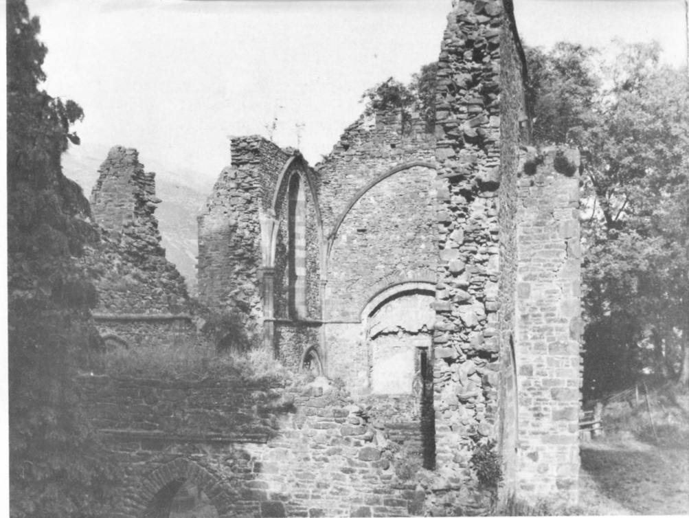
The need for urgent works to make safe the church walls is seen here
